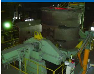
Ladle tilting unit
