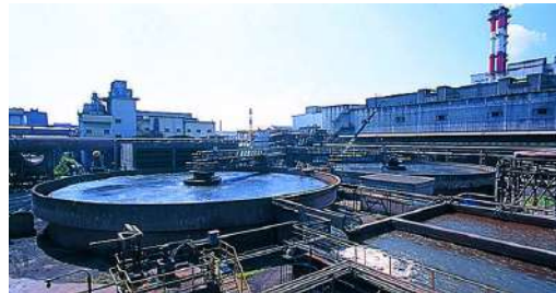
Industrial water treatment
